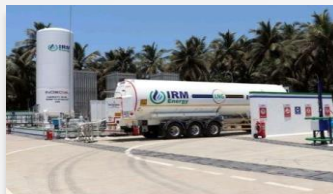
LCNG fuel station
